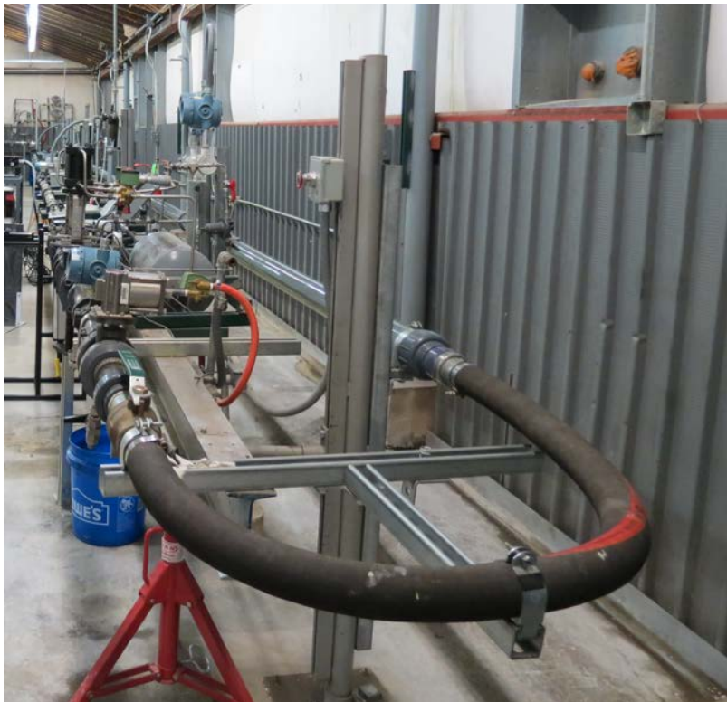
Figure 2. View of 2-in. High Viscosity Oil/Gas Two Phase Flow Loop
