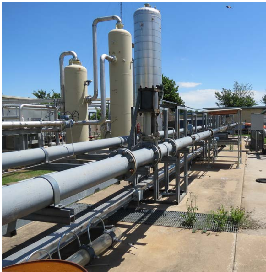
Figure 3: Side View of Low Pressure Large-Diameter Pipeline
