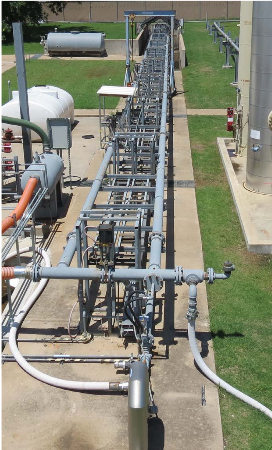
Figure 4: Top View of Low Pressure Large-Diameter Pipeline
