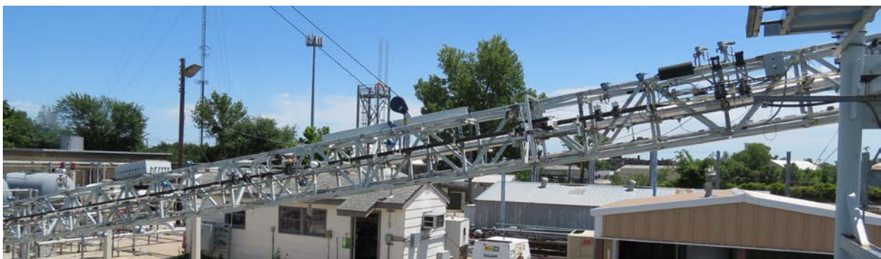
Figure 4. Close up view of the instrumentations at 2-in. Gas/Oil/Water Flow Loop
